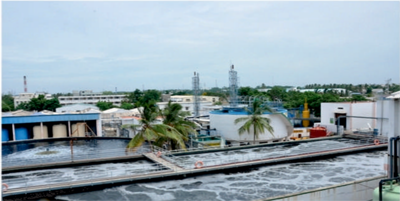
Effluent Treatment Tanks
