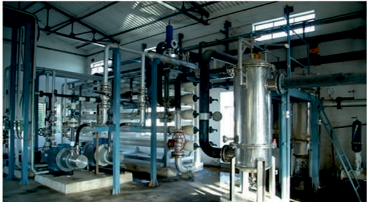
RO - Plant System
